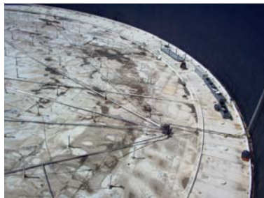
Temporary pipe lines on the floating roof
